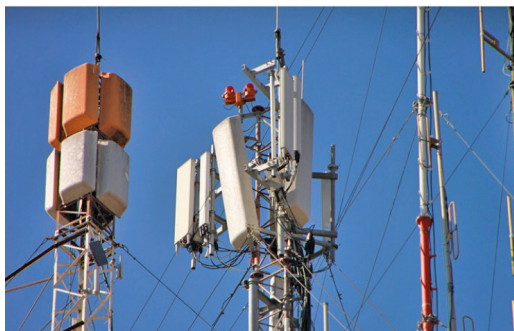
Figure 3. Base transceiver station (BTS)
